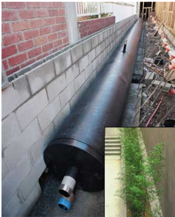
Rainwater cistern at NRDC's Santa Monica Office (inset photo after planter planting). Photo: NRDC.
